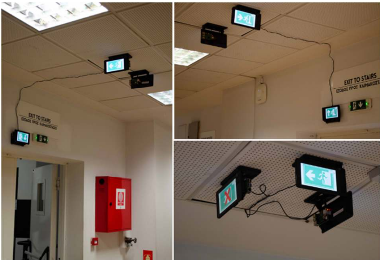
Figure 2: EVAGUIDE Exit signs installed at PAOK FC stadium in Thessaloniki during project pilot activities
